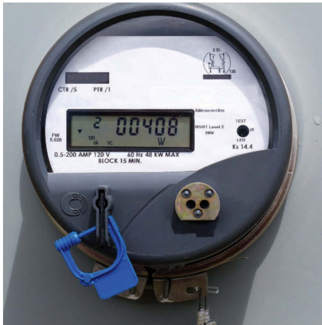
Figure 3.14 An example of a smart electricity meter.
