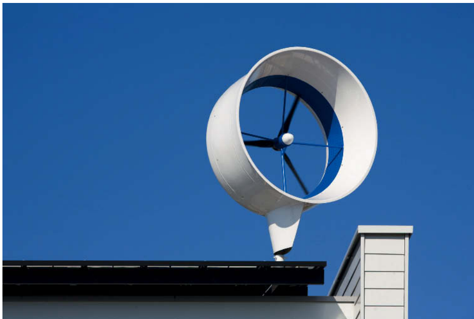
Figure 3.19 Small wind generator on a domestic property.
