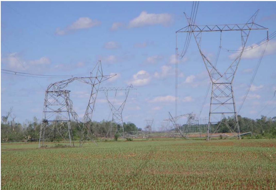
Figure 4. Damaged 500kV corridor near Athens, Alabama (courtesy of TVA)
