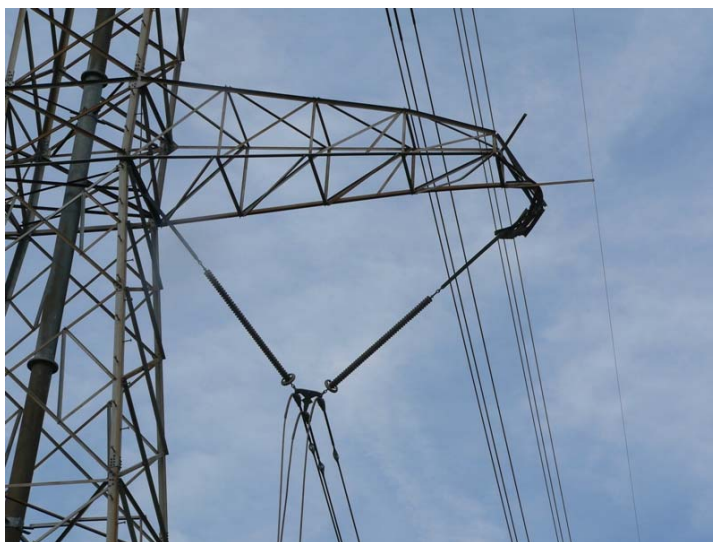
Figure 1. Arm Failure Due to Broken Conductor
