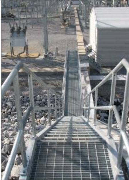
Photograph 8 Cable Tray on Stairway
