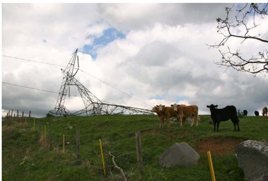
Figure 2 – Destroyed 500kV Tower
