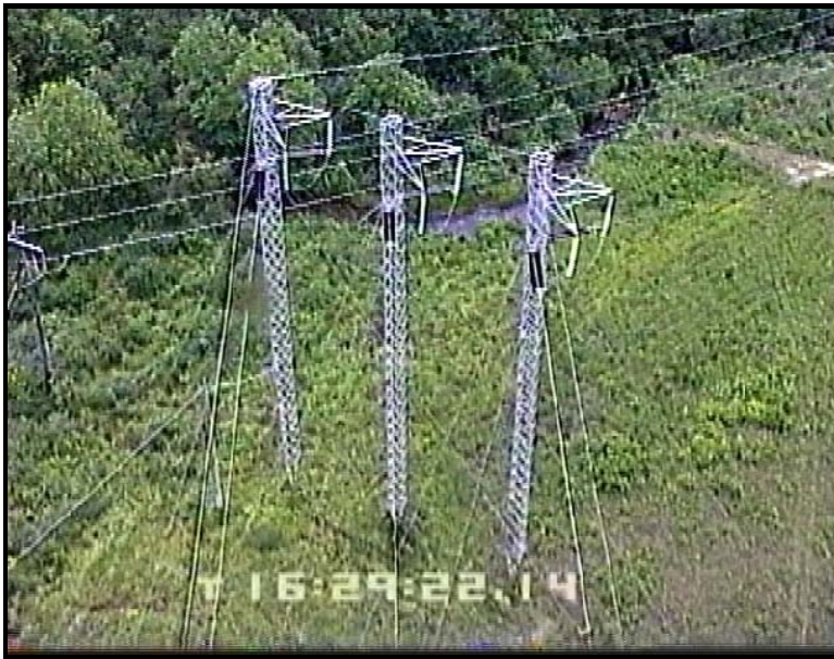
Photograph 1 - 230kV 3 Tower Aluminum Guyed Angle Structure
