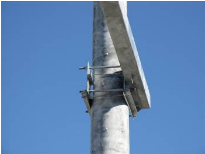
Photograph 7 Clamped Connection on Concrete Pole
