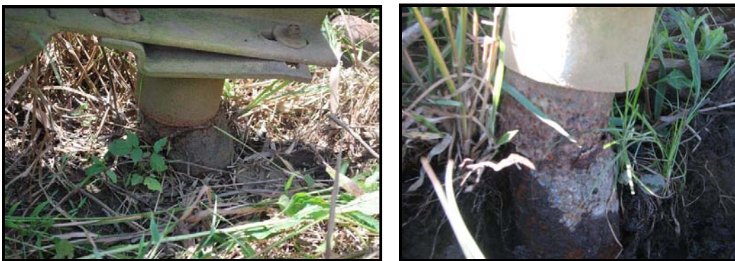
Photographs 3 and 4 – Severely Corroded Grillage Pipe Anchors
