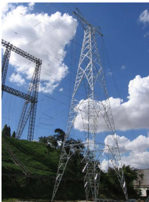
Figure 5: \pm 600 kV HVDC Self-supported Suspension Tower – Bipole 1
