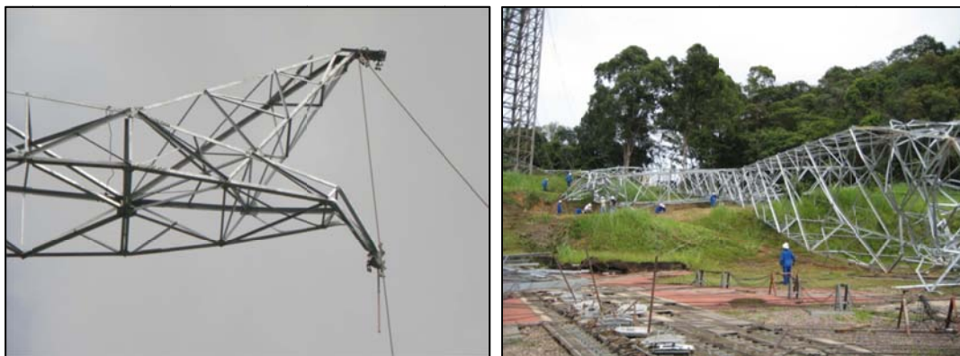
Figure 4. Tower D5A local arm failure and complete failure under 110% load.
