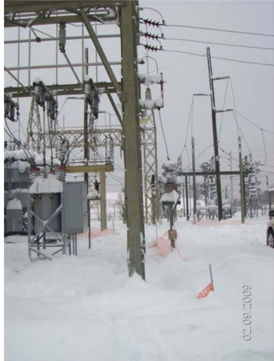
Photograph 2 – Two Foot Snowstorm at Whiteley Sub
