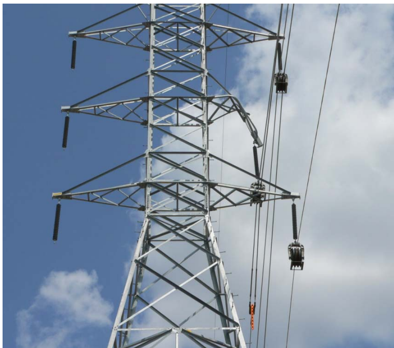
Figure 8. Longitudinal View of Arm Failure
