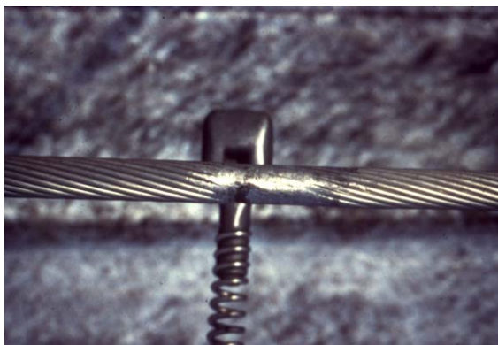
Figure 5a – Abrasion Damage at Spacer
