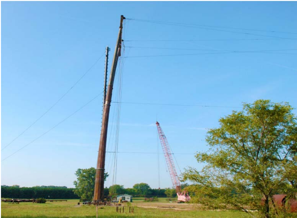
Figure 11 (Deflected Y-frame at 100% load increment)
