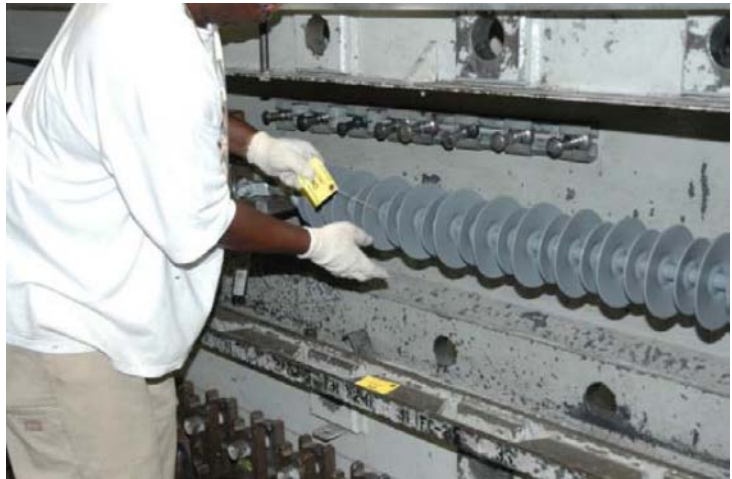
Figure 6 - Final check on a polymer insulator (Photo courtesy Southern California Edison)
