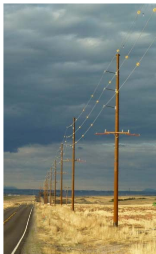
Figure 7. Spiral bird flight diverters (with permission from POWER Engineers).
