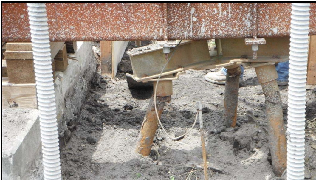
Photograph 14 – Middle Tower Exposed Grillage Foundation with Severely Corroded and Displaced Anchors
