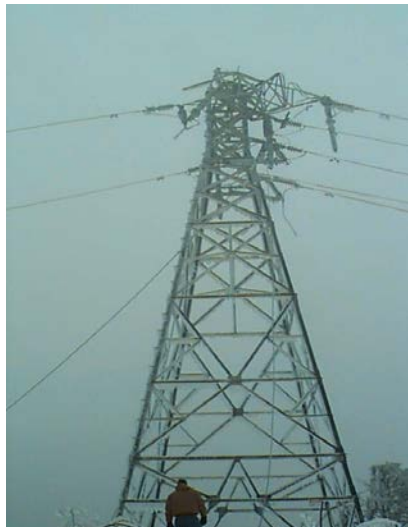
Figure 1 - 1998 tower failure due to extreme ice.
