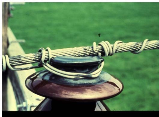
Figure 5b – Abrasion at Loose Hand Tie
