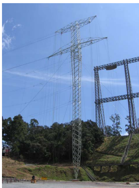
Figure 3: 2x500 kV Monomast Guyed Suspension Tower - Lot C
