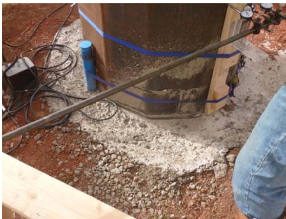
Photograph 3 – Tesla Slope Inclinometer Casing
