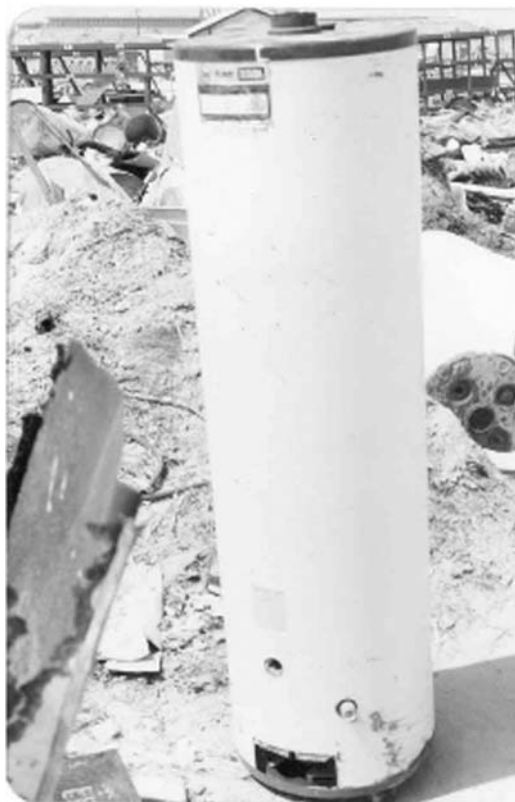
Figure 8.13 Initiation of corrosion of water heaters by ingress of moisture in insulation
