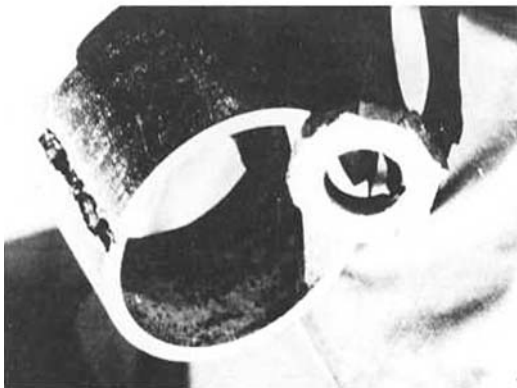
Figure 4.12 Graphite corrosion in gray iron pipe. (From Ports, R.D. (1987). Nalco Chemical Company)
