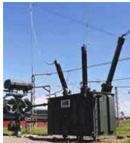
Shunt reactor, 400 kV, 150 MVar
