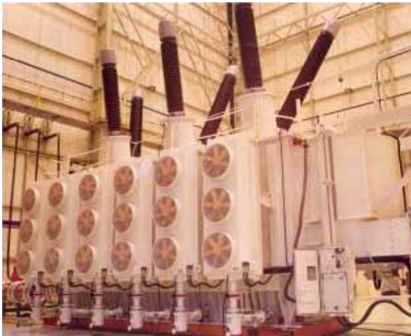
450 MVA auto-connected system intertie transformer
